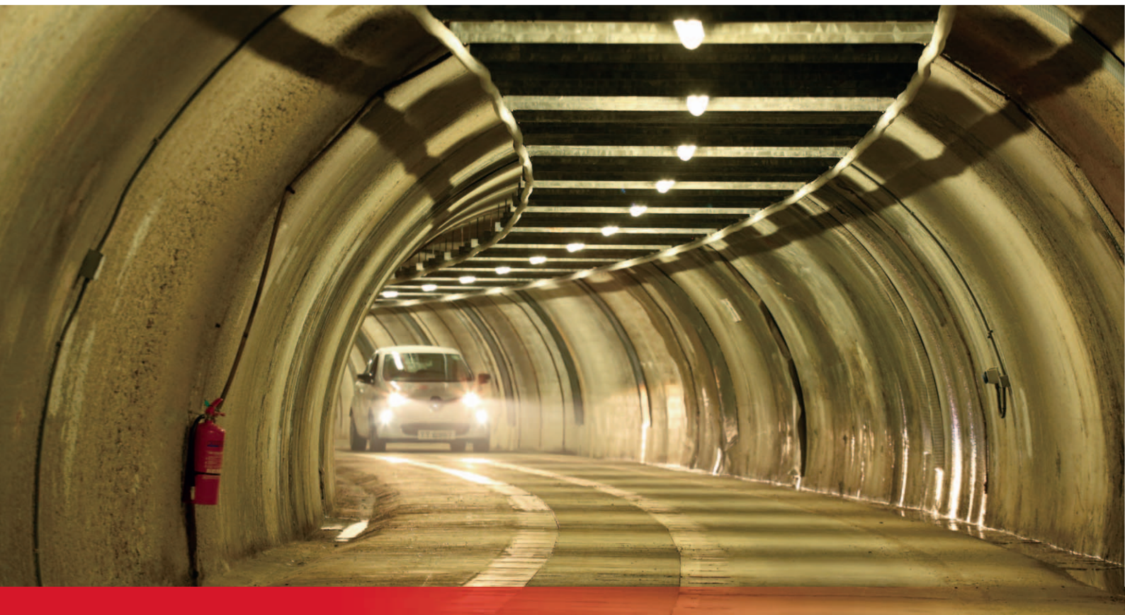
The Nam Fung Parker cable tunnel is one of the longest in the world at 5.7 km.
